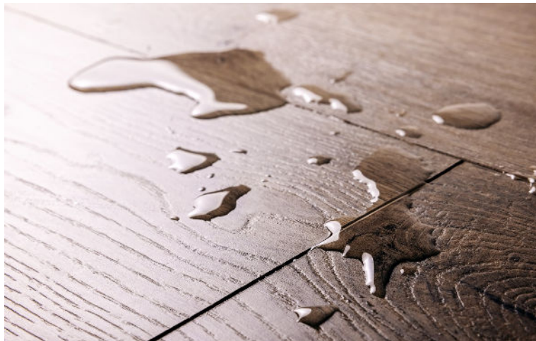
Figure 1: Spilled Water over a joint between laminate flooring
